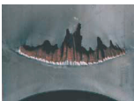
Fig 8 Close up view of damage caused by erosion on a gate valve
